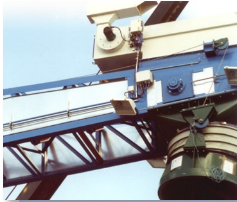
Cooper flange on a ship loading conveyor
