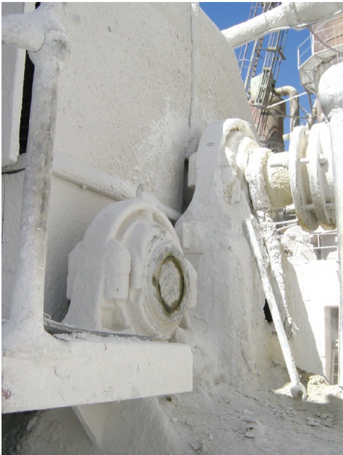
Bearings in a cement plant
