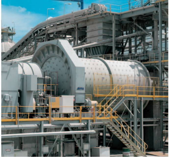
Figure 4 Bearing arrangements in comminution and processing plant
